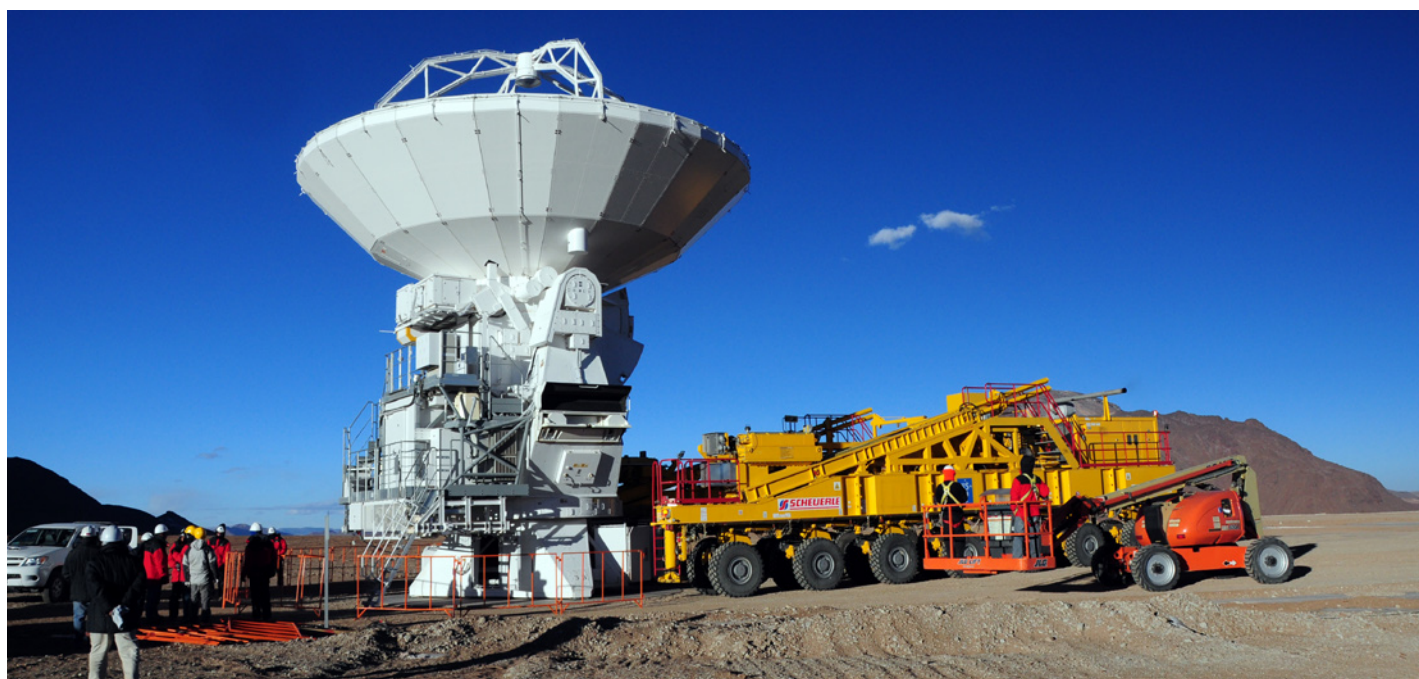
The transporter is shown in the process of setting the antenna down on the antenna foundation. On the right side is a manlift, which if needed, allows to access the surface and subreflector of the antenna.
