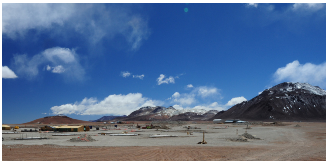
A photo of the work at the AOS site, at 5km elevation. In the foreground are antenna foundations for the Atacama Compact Array (ACA) for which the concrete pouring work is complete. For these, the power, signal connections and the antenna mounts must be installed. In the background is the AOS Technical Building.
