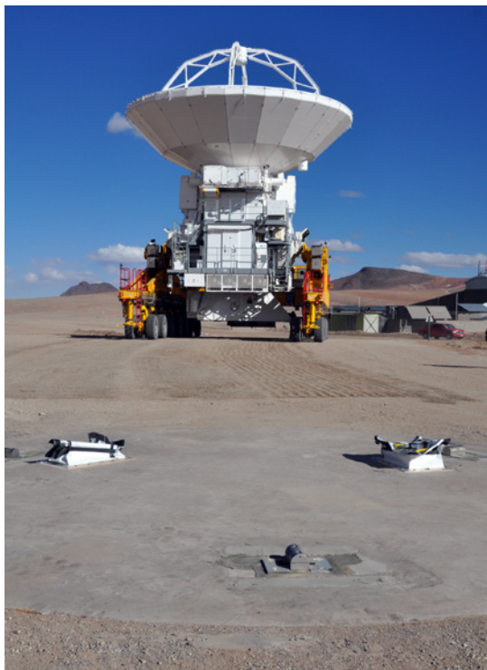
The transporter is shown carrying the antenna to the antenna foundation at the AOS
